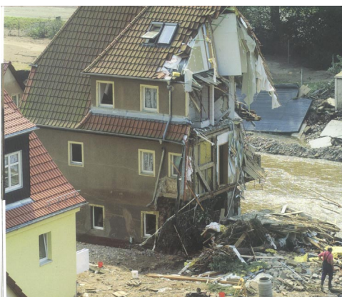
Photo 3 Failure of walls during the flood in August 2002 in Germany (Reimer, 2002)
