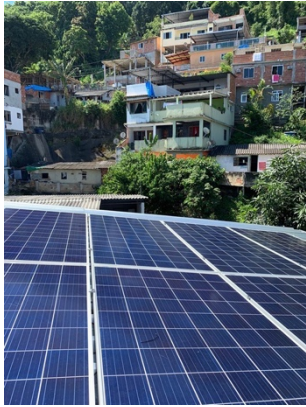
Figure 1-12 “ Babilônia Rio Hostel ” PV power plant (2016).
