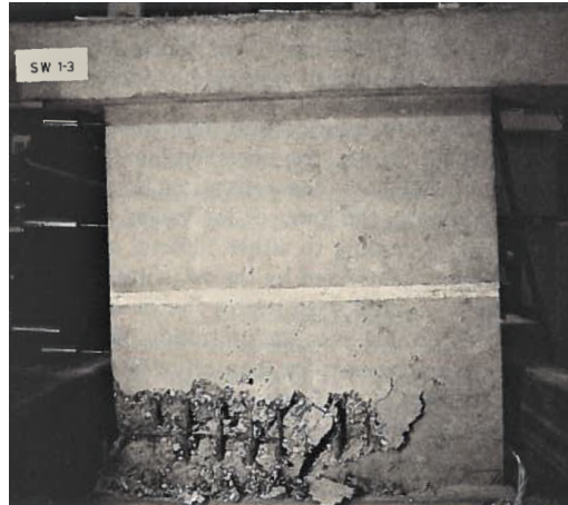
FIGURE 6.4: Wall SW13 at failure
