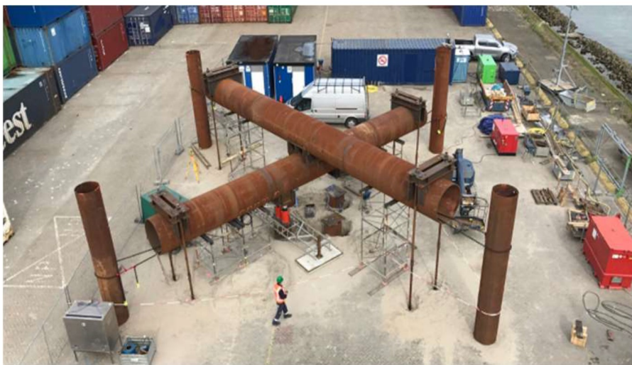
Figure 6.11: Load frame for pile load tests of 4 SI piles (Matic et al., 2019)
