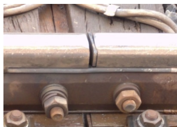
(j) IRJ number 16 with damaged insulation layer and a crack in the fastener.
