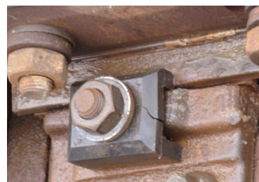
(k) IRJ number 16 with damaged insulation layer and a crack in the fastener.
