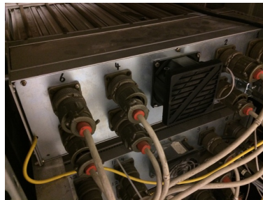
Figure B.14: 14: Two schematic lines wrapped in single cable housing at rear of Ch. 4 signal conditioner
