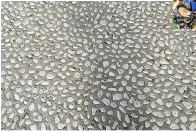
concrete structure mixed with pebbles and demolition material
