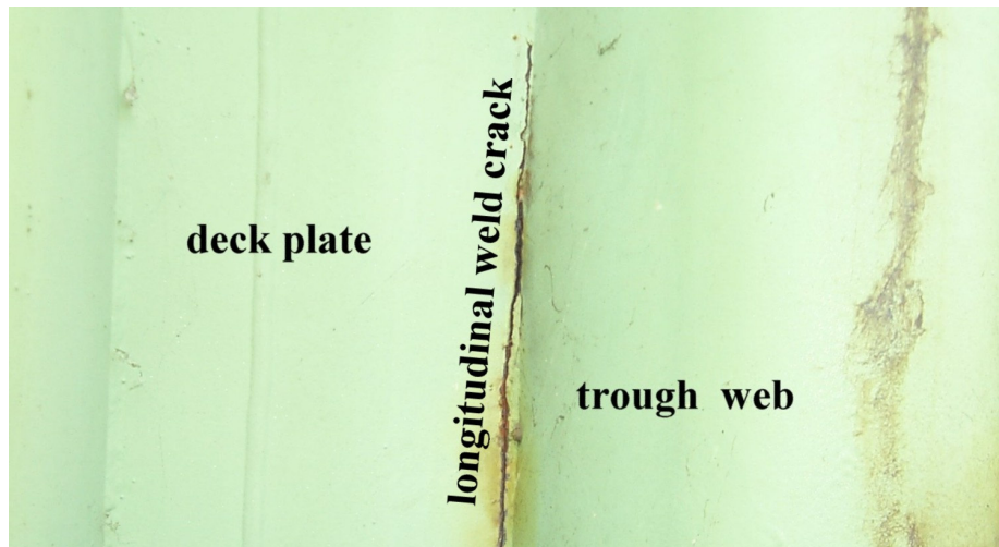
Figure 2-17: Visual observation crack in the longitudinal weld trough – deck plate
