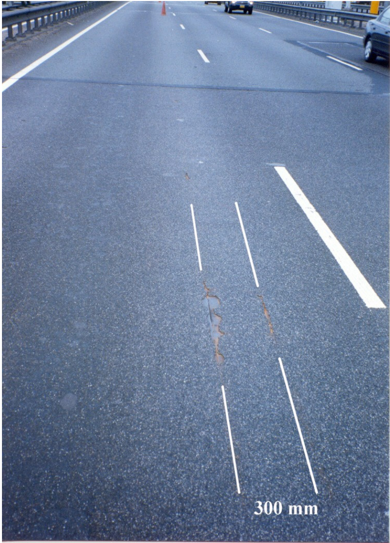
Figure 2-11: Visual observation of deck plate cracks in movable bridge
