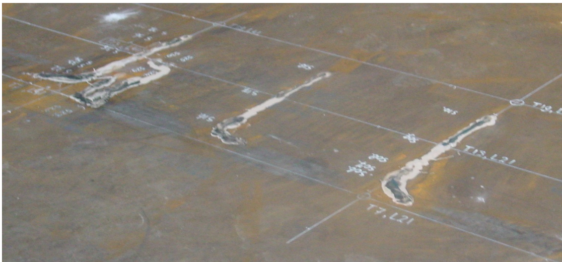
Figure 4-56: Protection of strain gauges on top of steel deck plate, section 1, locations 1 to 5
