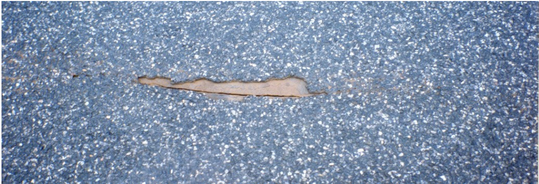
Figure 2-12: Detail visual observation of deck plate crack in movable bridge
