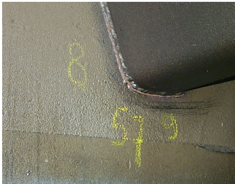
Figure 2-24: Visual observed fatigue crack trough – crossbeam connection
