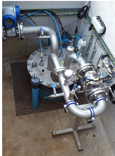
Figure 2.3: Top of the Smart Well
