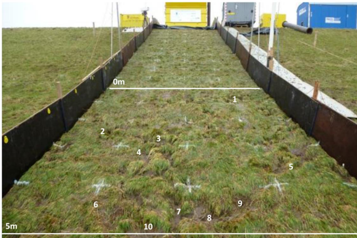
Figure 46 - Example of various bald spots during wave overtopping tests in Millingen aan de Rijn (Infram 2013)
