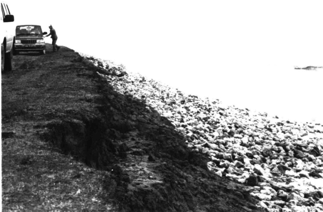
Picture I.5 Damage on stone revetment in Hai Hau District
