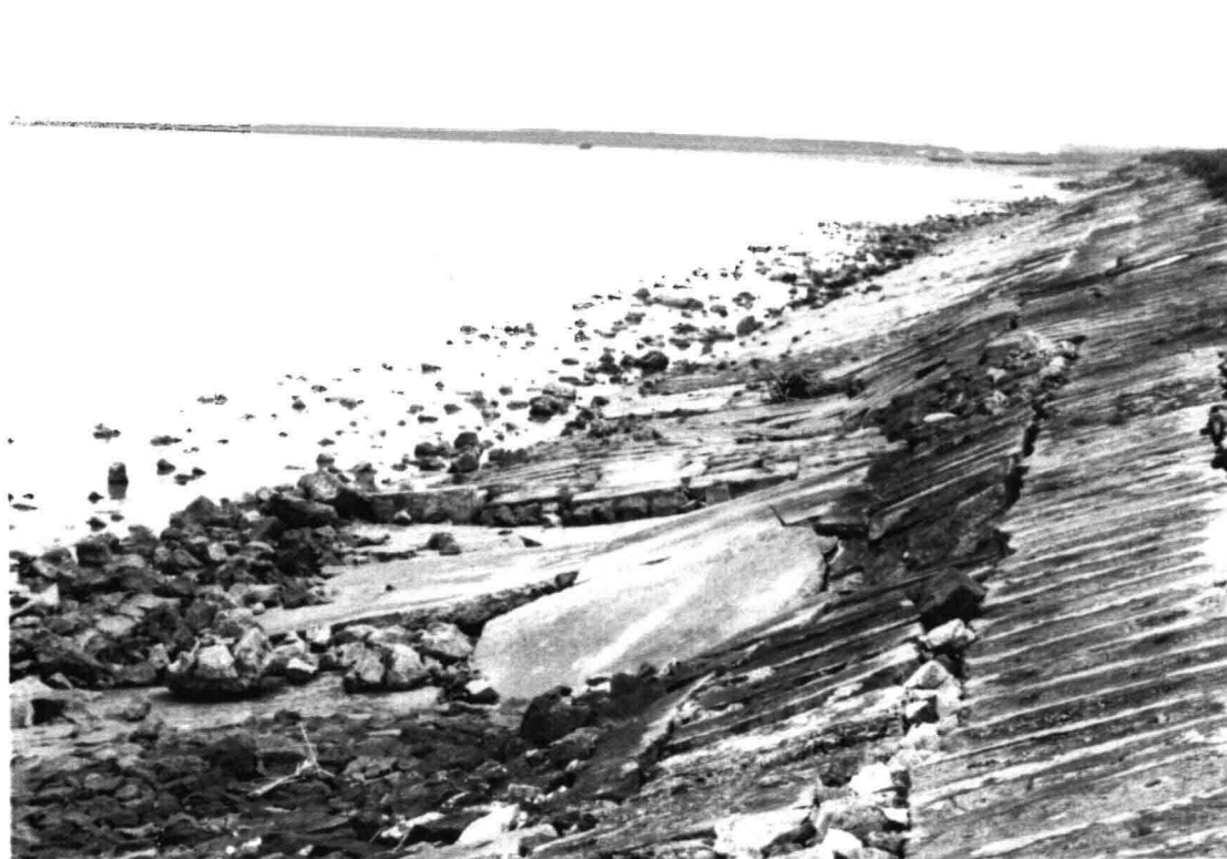
Picture I.7 Damage of concrete grouted stones revetment in Hai Phong Province
