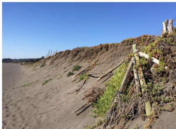
Figure 5.23: Picture of the steep interface between the beach and the dunes taken by the project team during the site visit of Pichilemu
