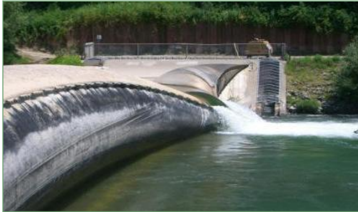
Figure 30: An inflatable dam with a 'V-notch'.
