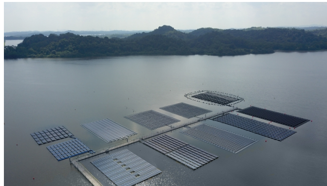
Figure 2.2: An example of a floating solar installation on water in Singapore [11]
