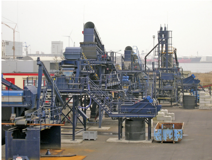
Figure 1.5: Pilot plant for wet physical separation of BA with a capacity of 50 t/h.
