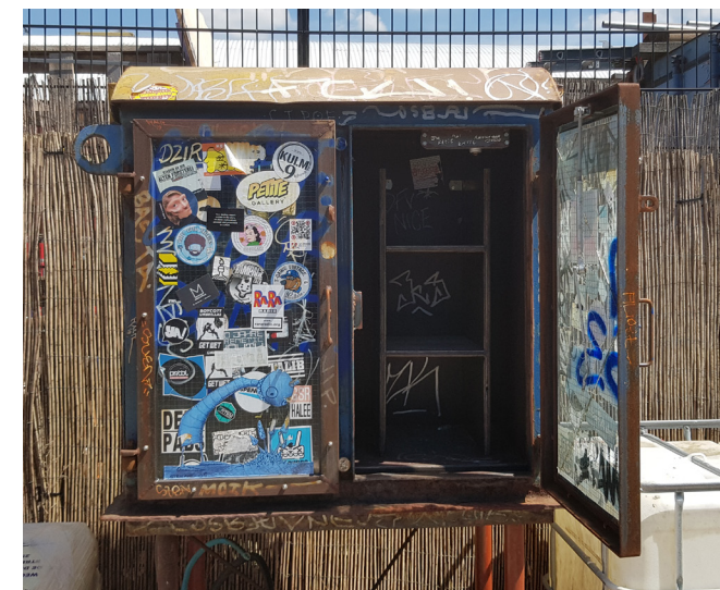
Figure 5.2.3, Cabinet at NDSM-wharf
