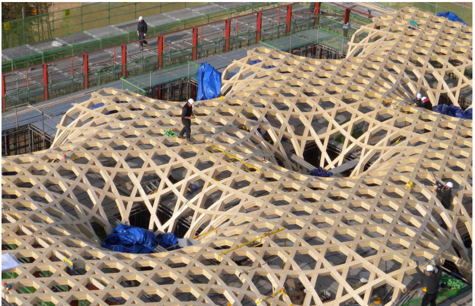
Figure 11 Detail view of the timber roof nodes at the Haesley Nine Bridges Golf Clubhouse from Haesley Nine Bridges Golf Clubhouse, Yeosu - Shigeru Ban, by Arquitectura Viva, 2021, ( https://arquitecturaviva.com/works/club-de-golf-haesley-nine-bridges-0# ).
