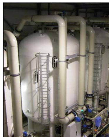
Figure 7: Softener at DWPB (Evides Industriewater).
