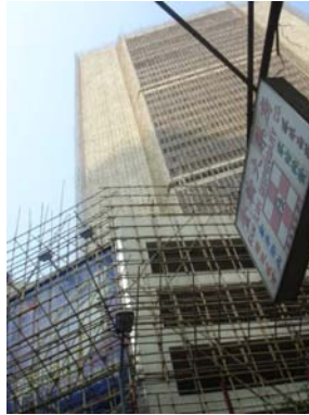
Figure 9.17: In Asia the bamboo stem is commonly used in scaffolding, even for the construction of skyscrapers
