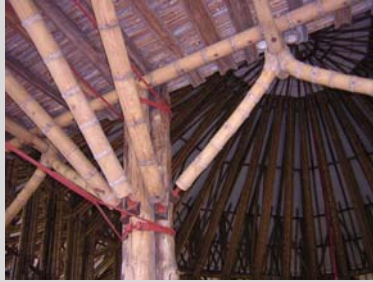
Figure 9.13: The Colombian architect Simon Vélez fills the final chambers of bamboo with concrete to create a stronger connection with protruding bolts
