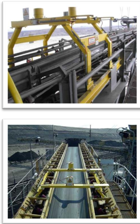
Figure 2.6: Radiometric sensor measurement device, installed on the conveyor belt, measuring blend of coal resulting from multiple excavators, just before the stock Pile (Source: MIBRAG)
