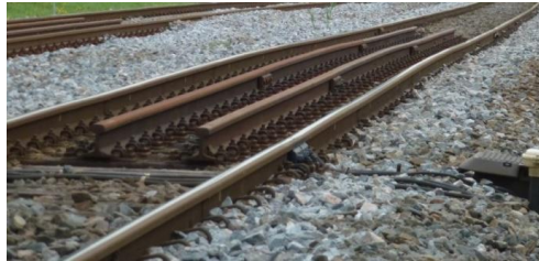
Figure 4.3. Transition zone with a large differential settlement.
