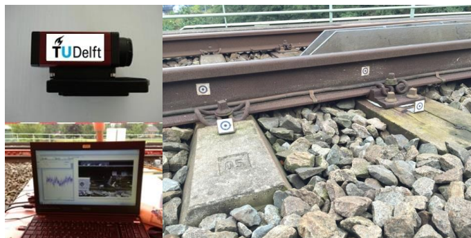
Figure 4. Setting of DIC-device: high-speed camera, software and targets on rails and sleepers.
