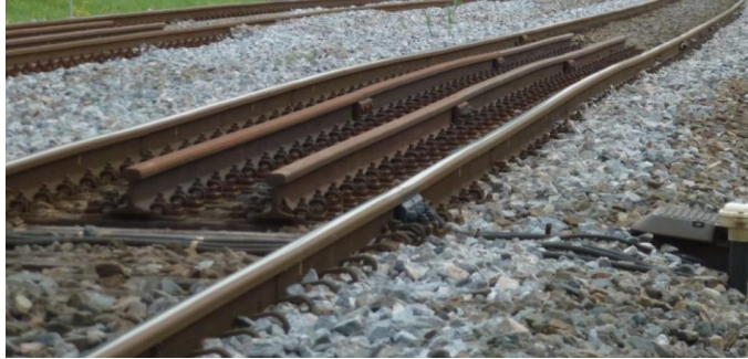
Figure 2.2. Track settlement in the transition zone.
