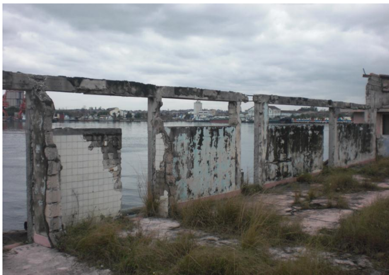
figure F.8 – the current state of a part of the Muelle de la Coubre (03/02/2013)
