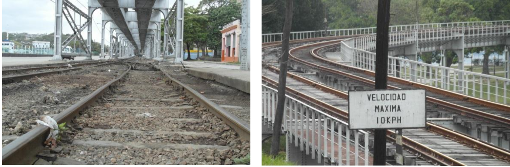
figure E.41 – bad condition of the rails (left) and low speed (right)
