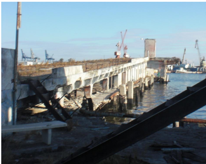
figure F.7 – the dilapidated state of Espigón del Vaciadero (02/09/2013)
