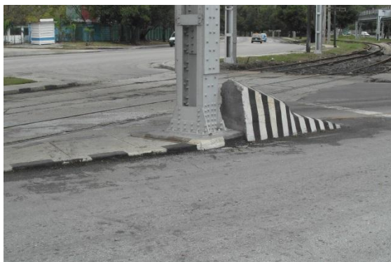
figure E.43 – marked column at the intersection between Avenida del Puerto and Arroyo
