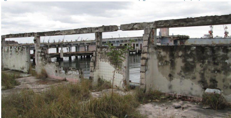
figure F.19 – the remains of structures on the Muelle de la Coubre (03/02/2013)
