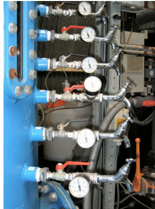
Figure 4.3: Plug valves and pressure gauges installed along the filter bed of the pilot scale dual media filter at WWTP Horstermeer
