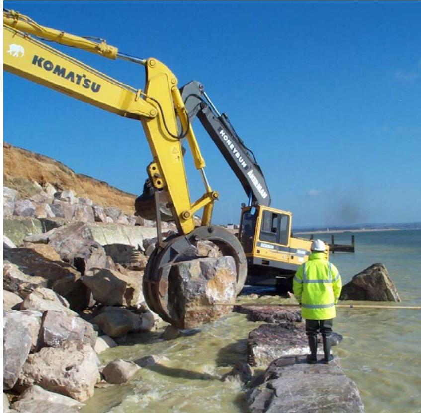
Construction continuing on a rising tide following placement of the ‘toe stones’
