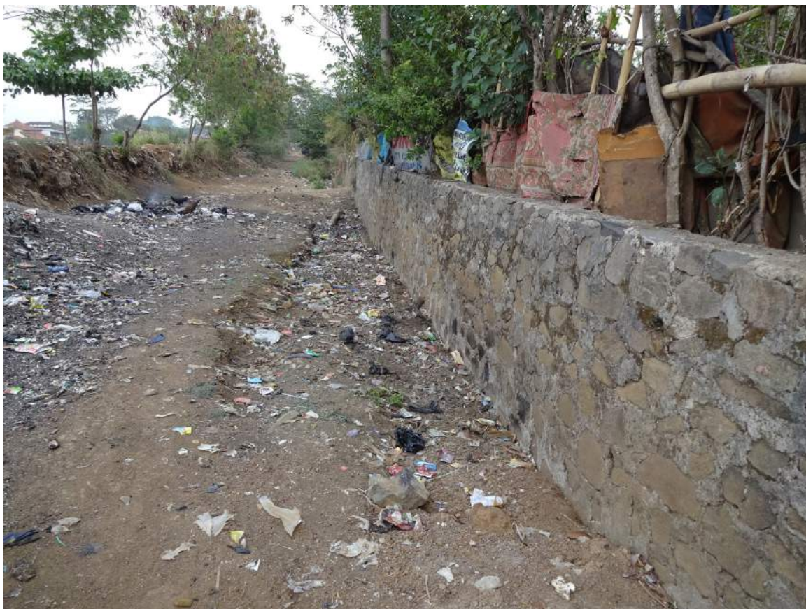
Figure 42 Condition of the inspection road and drain. Dayeuhkolot Village Source: Author
