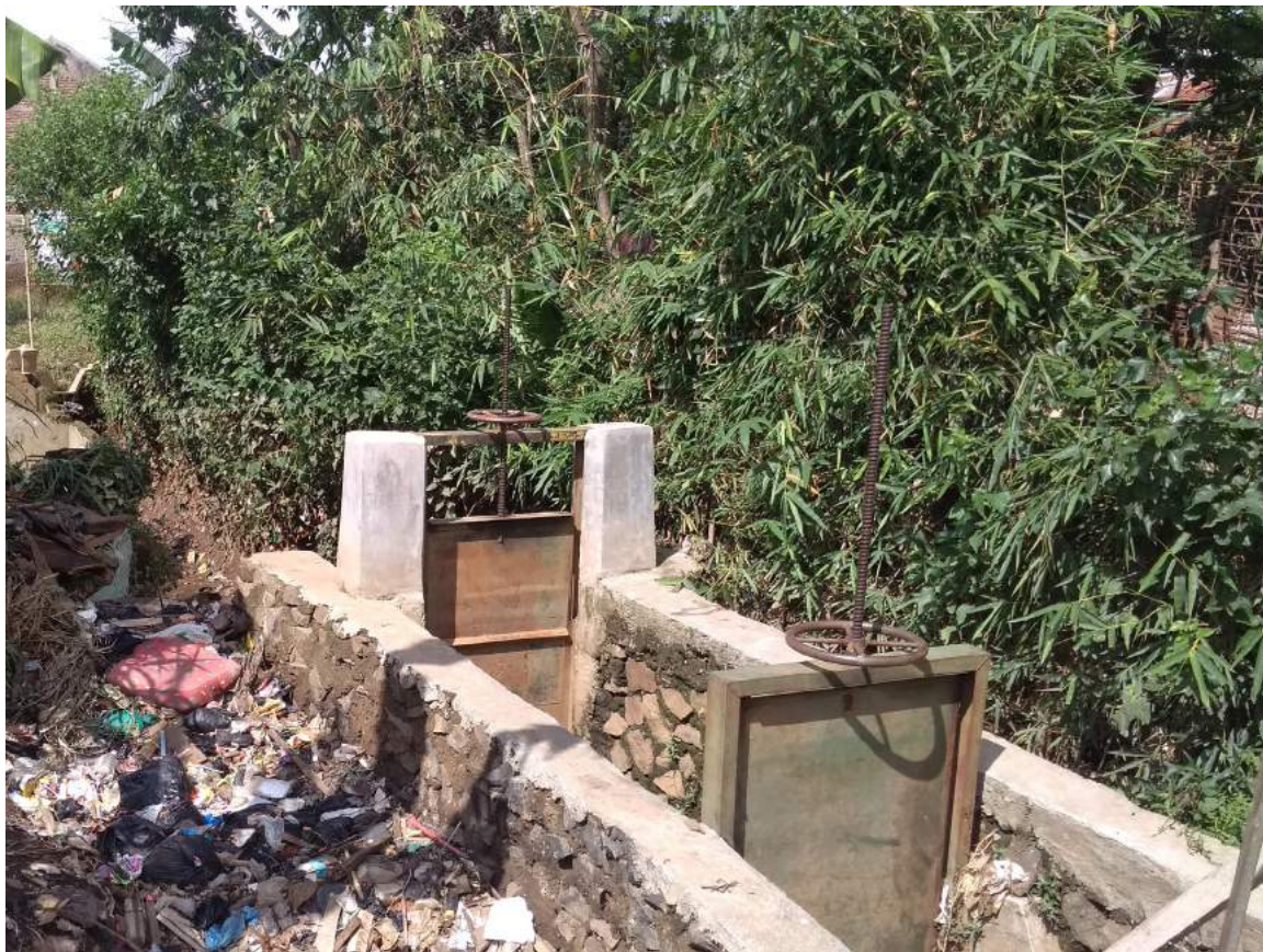
Figure 43 Water Gates installed for protection from solid waste entering the area during flood events Source: Martin Muljana
