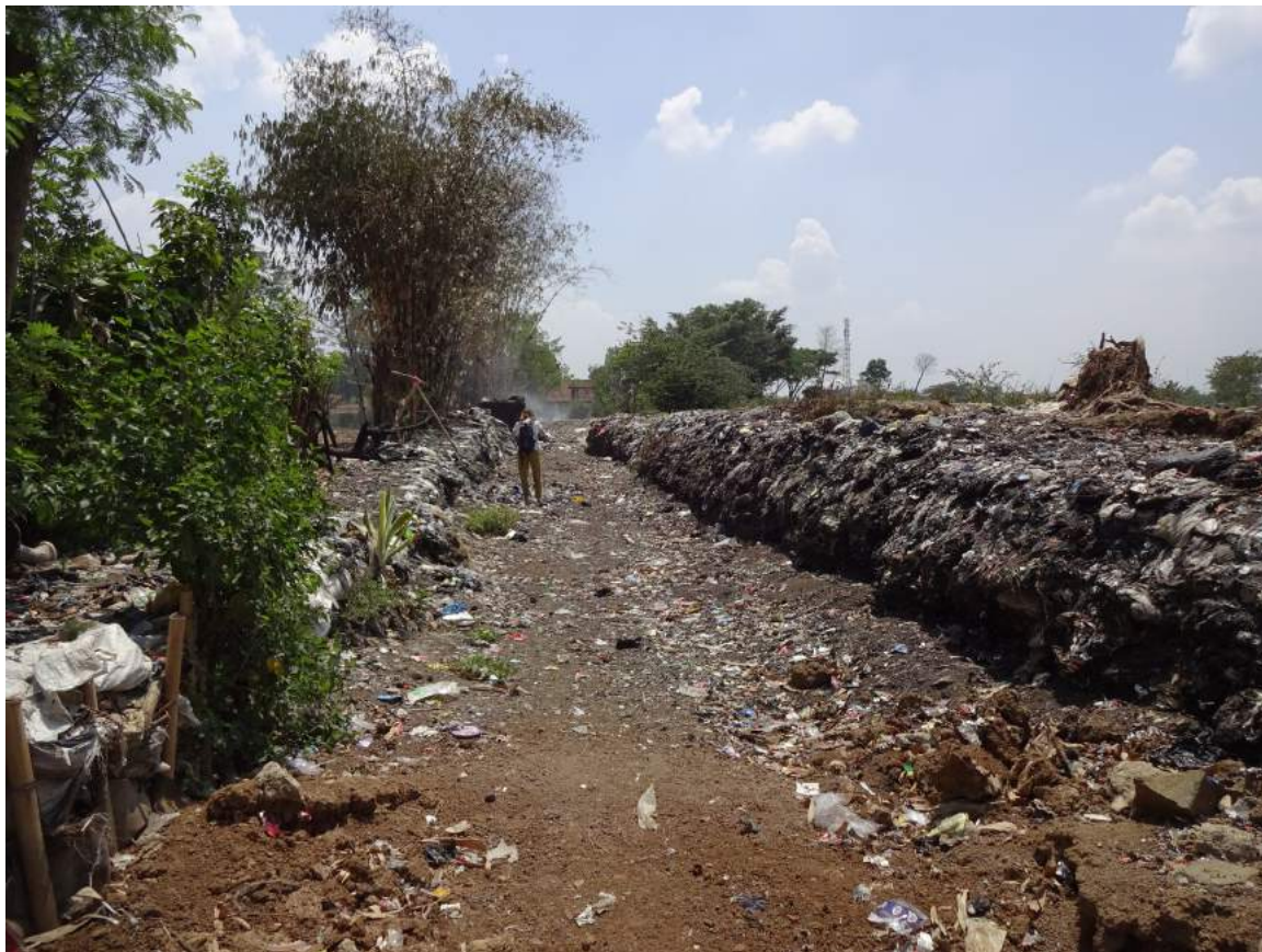
Figure 41 Existing dike near Dayeuhkolot Village - hight and condition of the soil Source: Author
