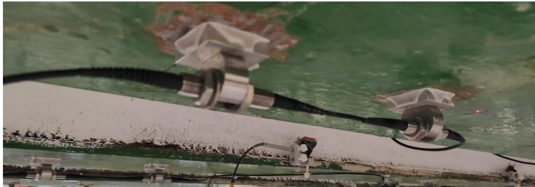
Fig.2.27. Fiber optic glued to the bottom of a steel beam.
