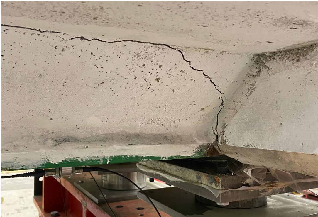
Fig.3.17. LB1. Crack from the east support along beam 1.
