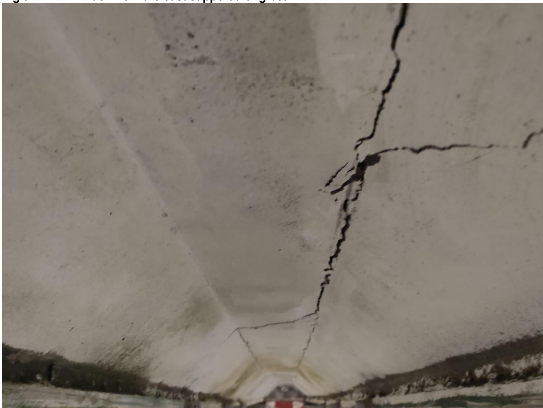
Fig.3.18. LB1. Crack between beam 1 and 2 underneath the specimen. The crack was observed after the test.
