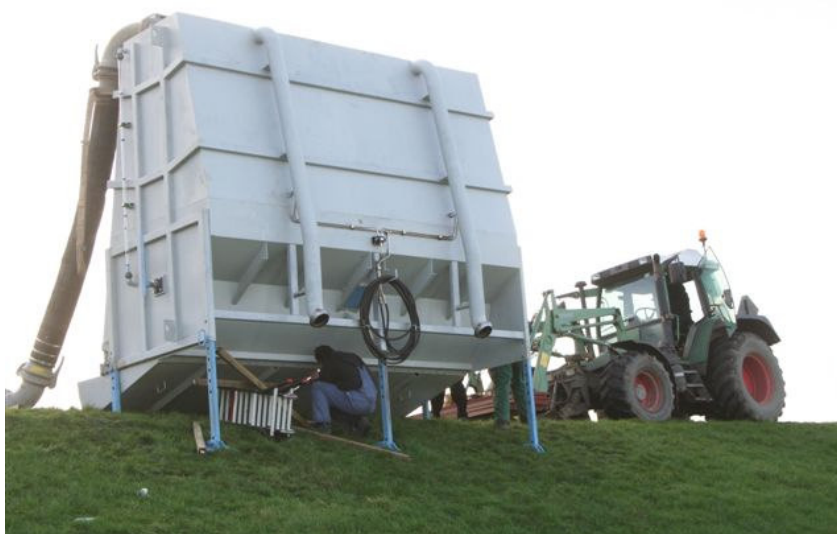
Picture 7.13. Installation on dike for calibration day and mounting of transition slope.
