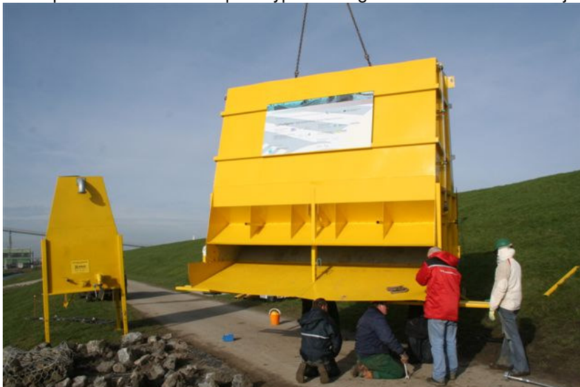
Picture 8.2. Mounting the transition or guiding slope onto the simulator while hanging in the crane.
