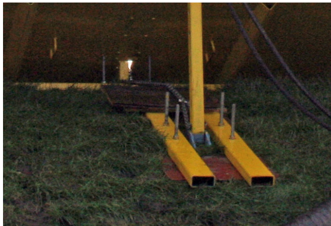
Picture 8.5. Detail of adjusted leg with extra steel girders and wooden plates.
