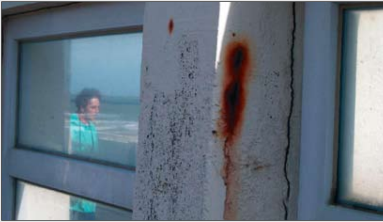
Another example at Blankenberge Pier. If in a saline environment like this, concrete damage is repaired with coatings alone, i.e. without using cathodic protection, the corrosion processes will return time and again.
