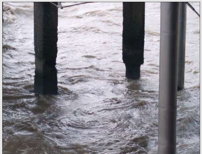
Heavily affected supports under the pier at Blankenberge (Belgium), a typical example of what happens if concrete is left unprotected.
