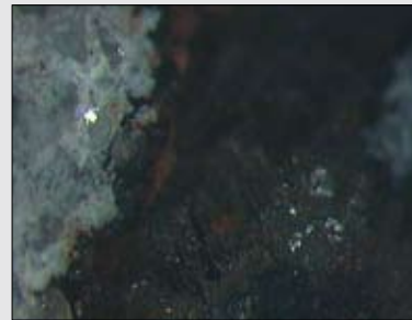
Steel pushed to corrosion, but now with cathodic protection.
