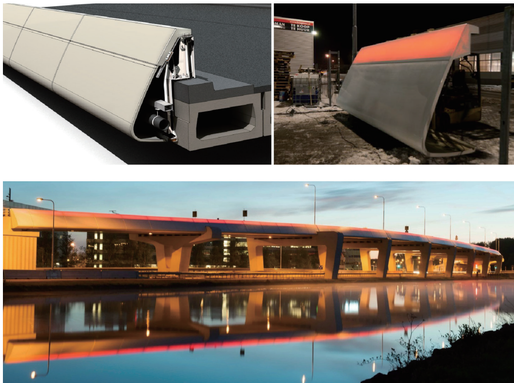
Fig. 10. Installation of red light in the panels of the highway N201 viaducts.
