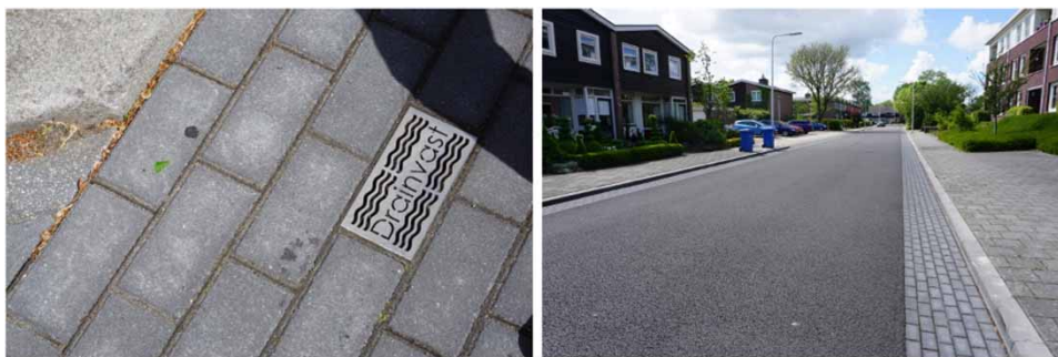
Figure 6 | Case #33 has been assigned the root cause Incomplete knowledge about the internal technical processes. The pavers were separated by joints filled with a permeable material, allowing water to infiltrate. Even after a small rainfall event, however, water remained ponding for at least 1 h. As such, it was thought that the permeable material had become clogged, leading to a malfunction of the SUDS.
