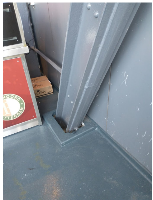
(f) A member going through a gap in a balcony
