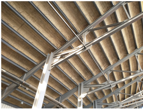
(c) Connection between the N-structure and the beam with the varying profile
