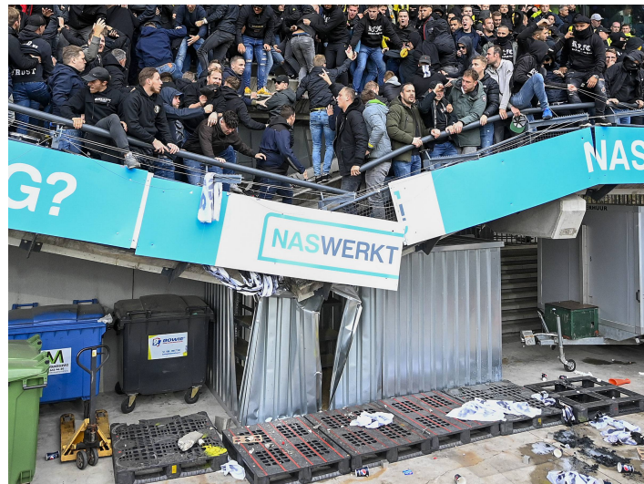
Figure 2.10: The collapsed grandstand element at De Goffert, from (NOS, 2021)
