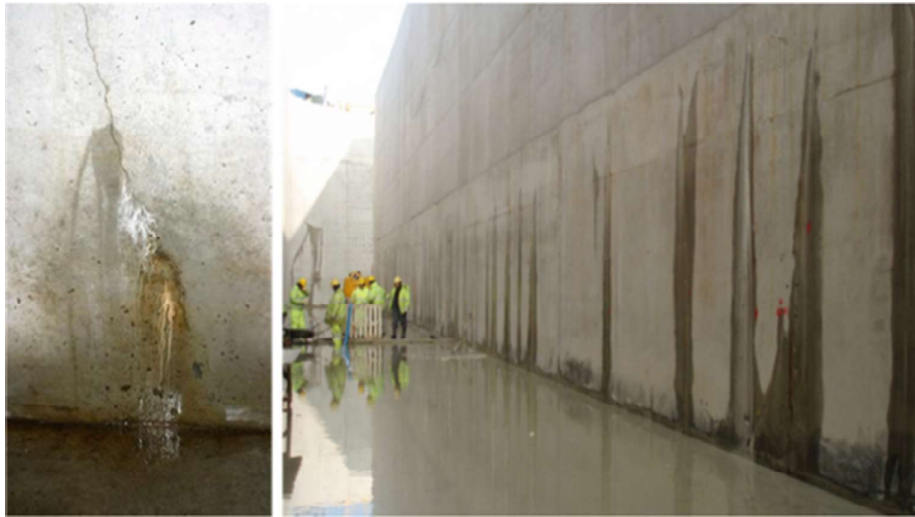
Fig. 1. Water leakage through vertical early age cracks in a wall-slab connection.
