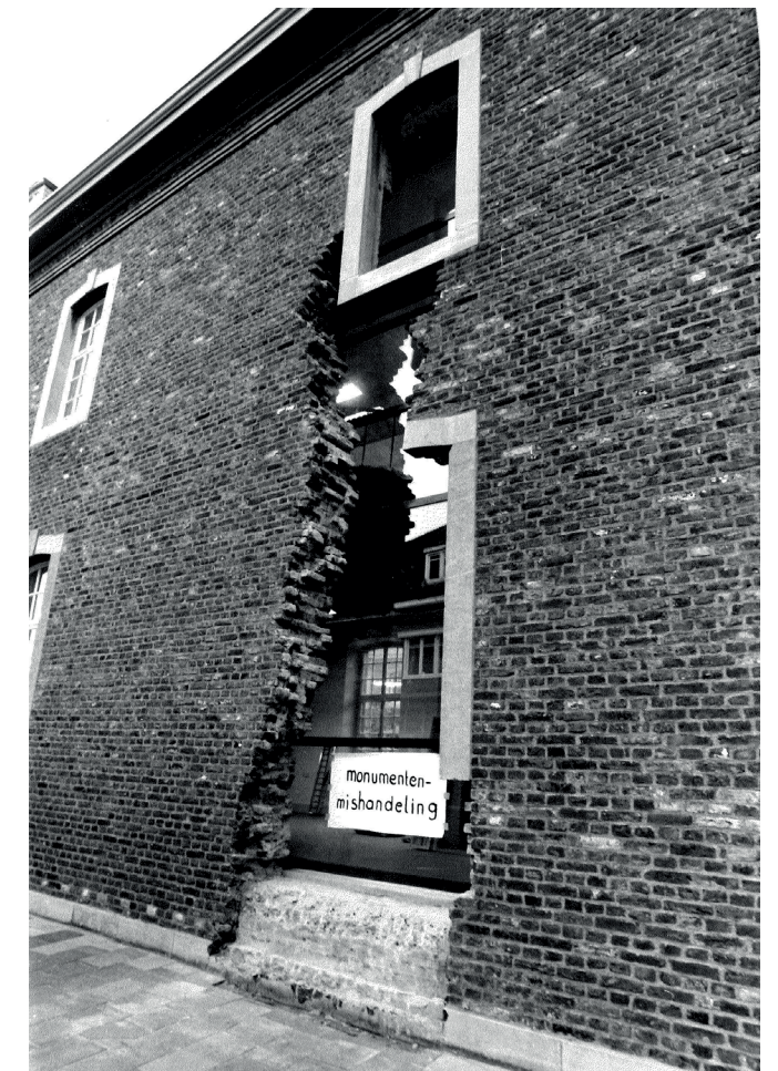
Figure 18. Crack with pamphlet of 'monument abuse' (RHCL, 1994)
