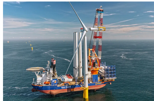
(b) The third, and last, blade of a wind turbine is being installed (Van Oord, 2020)
