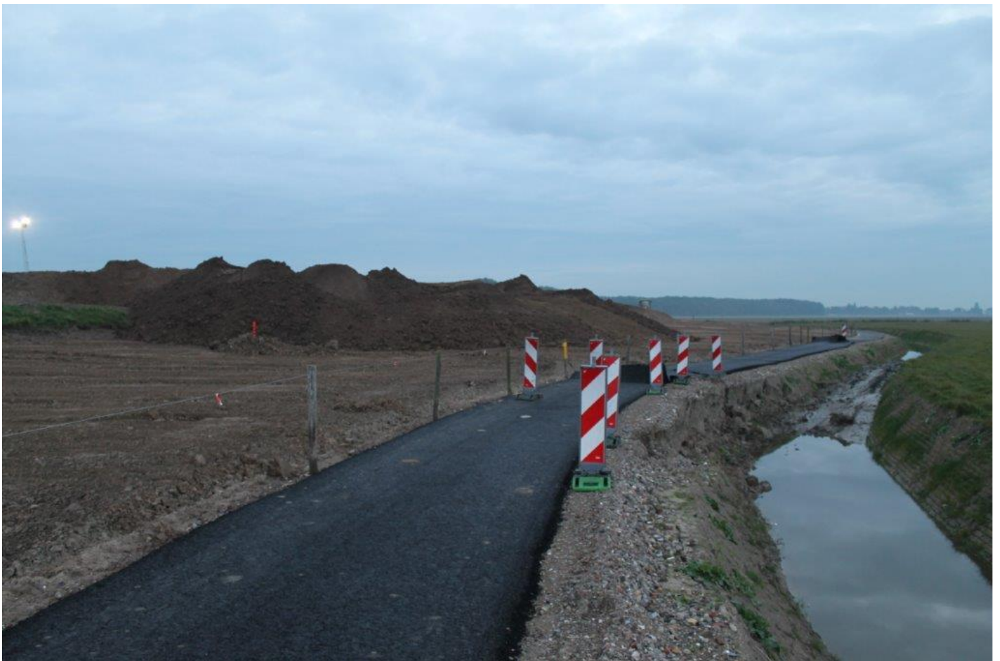
Figure 36. Overview of Shear and Clay Depot
