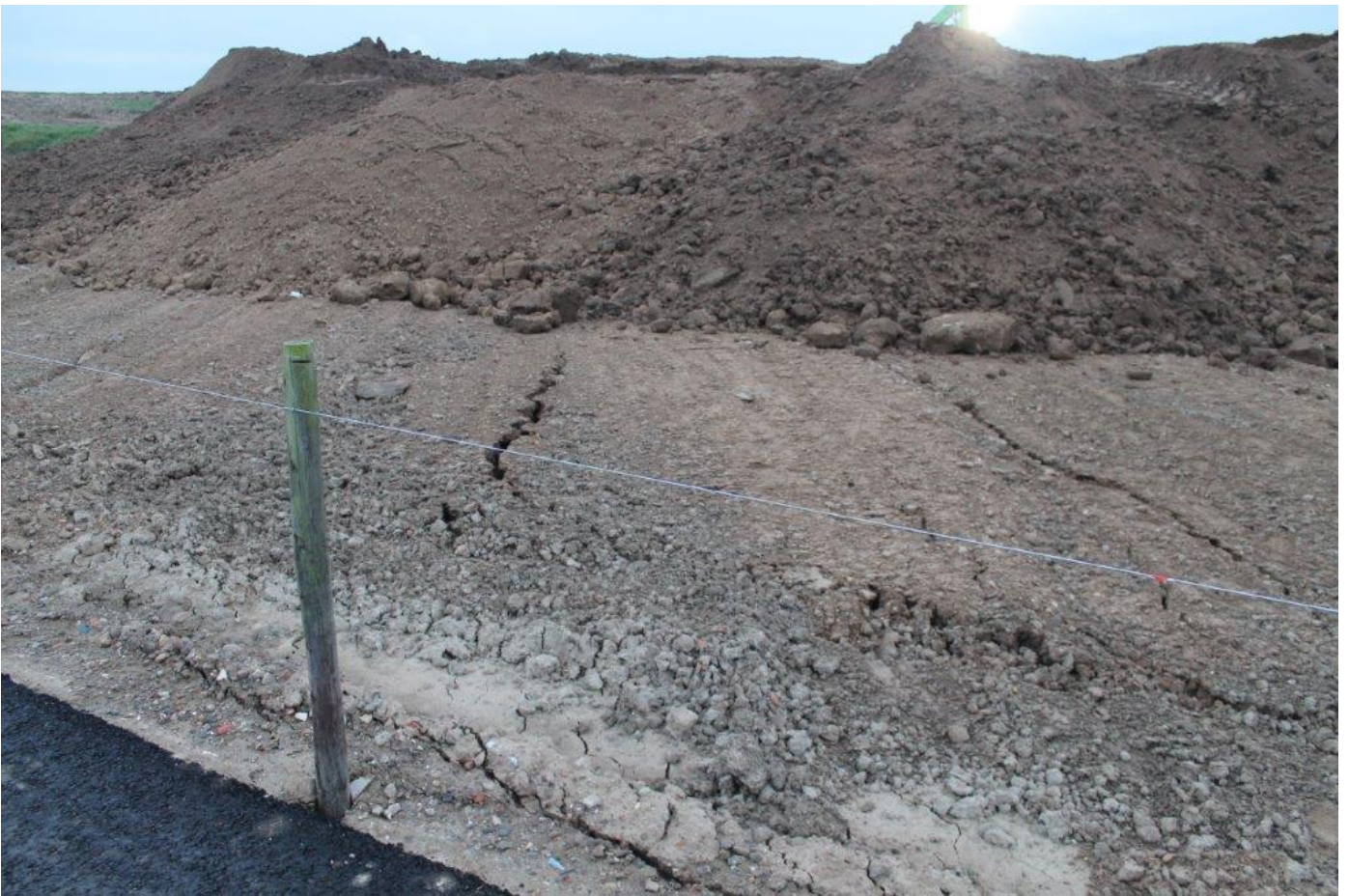
Figure 37. Shearing at Road Side
