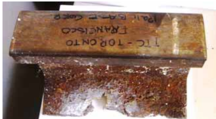
Figure 2.4: View of a section of 115-lb rail showing severe corrosion at the base of the rail [88].
