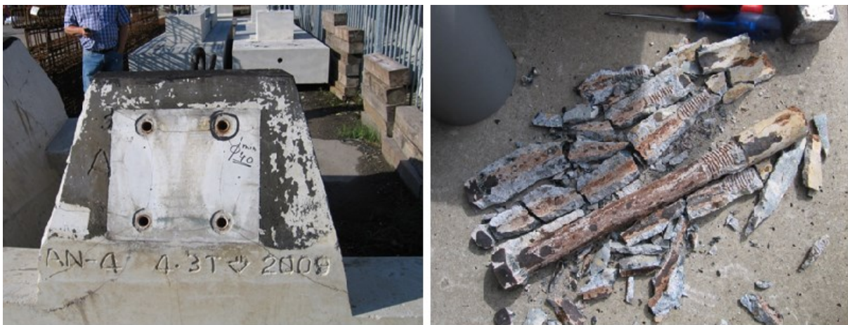
Figure 2.7: Damaged block due to the corrosion of anchor induced by stray current [105].
