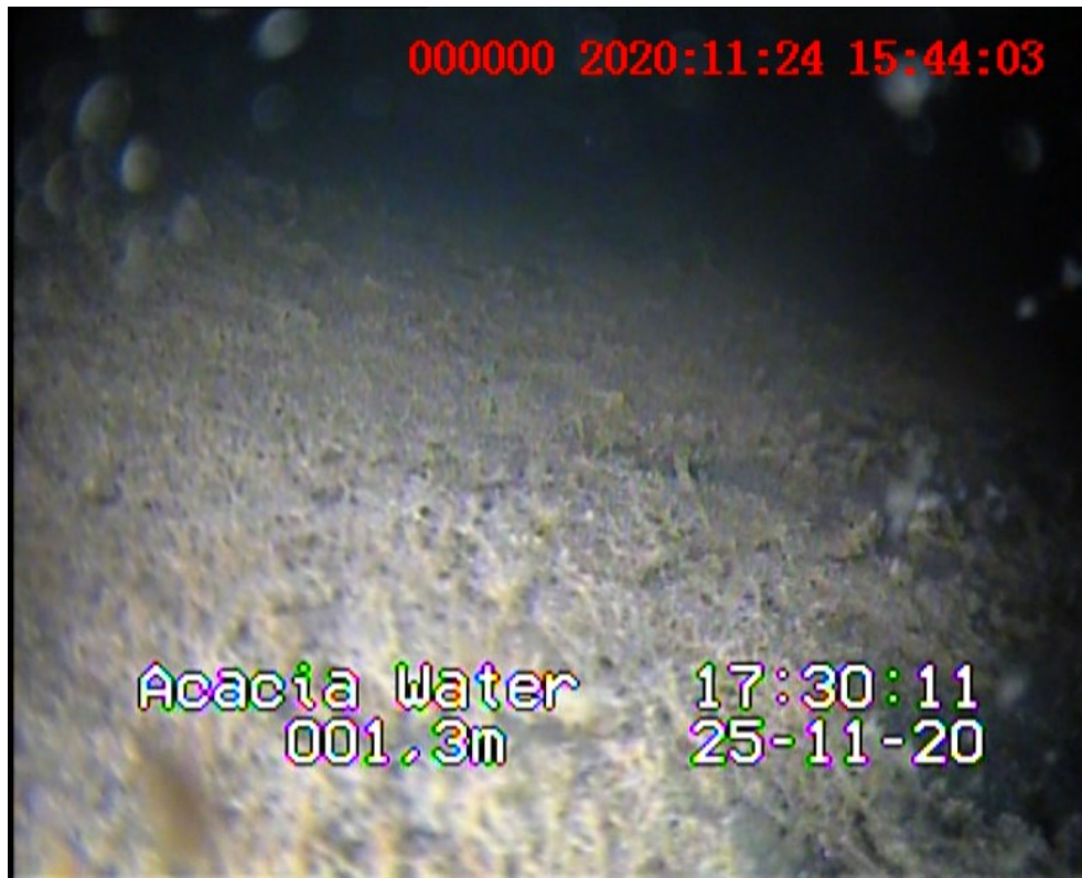
Figure 5.5: Camera shot of the conditions within the main tile outlet discharging tile drainage water to the drain reservoir. A mat of microbial deposits similar to that in the standpipe (fig. 5.3) is seen.
