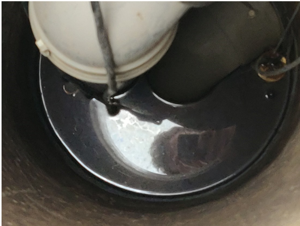
Figure 5.1: Metallic sheen on stagnant water within the standpipe taken November 25 th , 2020 after a 41-day standstill.
