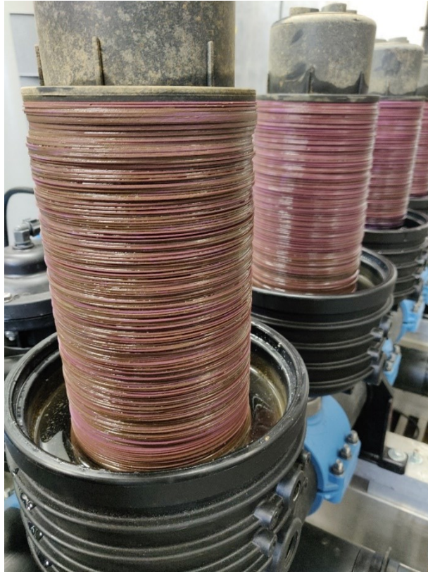
Figure 5.6: Image taken of the disc-filters after the head is removed. The filter is covered in brown slimy material. Shot taken November 25 th , 2020 after a 41-day standstill.
