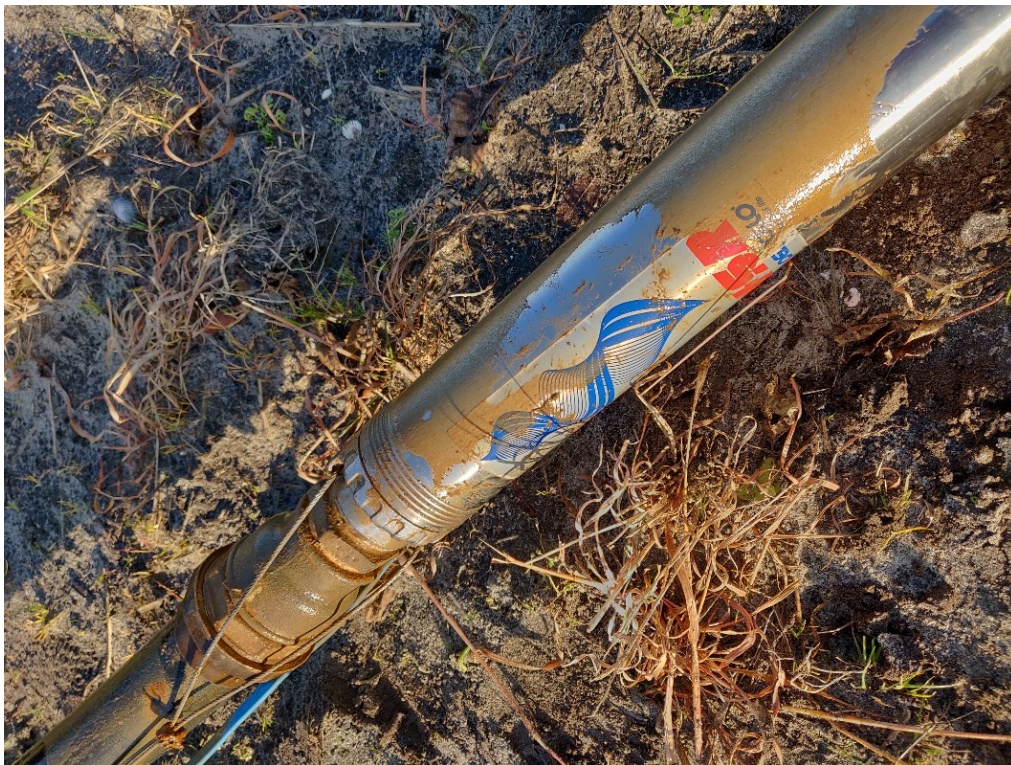
Figure 5.7: The automated backflush pump removed prior to the well rehabilitation on November 25 th , 2020. A thin layer of brown glutinous material is discerned suggesting iron oxides.
