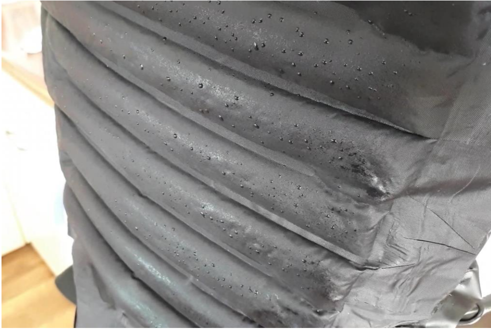
Figure 166: Condensation on the pad
