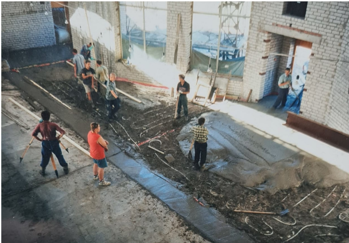
Fig. 13: Construction process of St. Paul Church. Visaginas museum archive. Author Jonas Danauskas, 1992.
