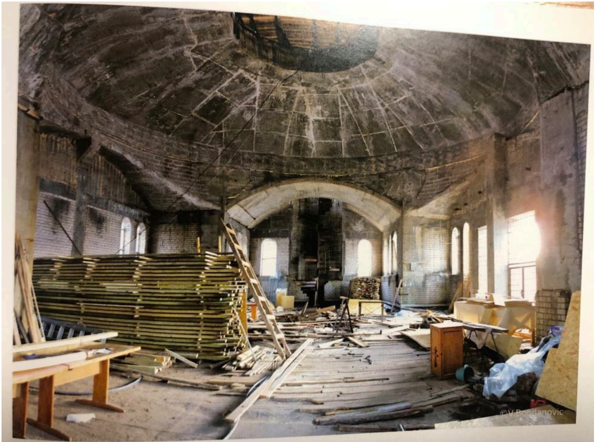
Fig. 24: Archival photograph of the construction process of Visaginas St. Martyr Panteleimono Church. Archives of Visaginas St. Martyr Panteleimono Church, 2006.
