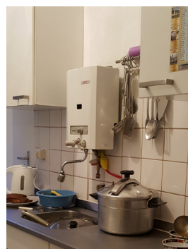
Fig. 1.2.7: Family: Gasboiler (open geiser)
