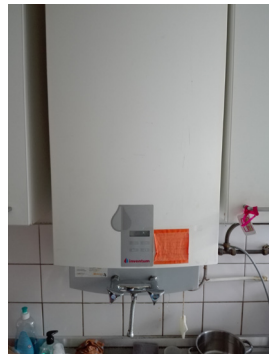
Fig. 1.2.2: Student 1: Gas boiler
