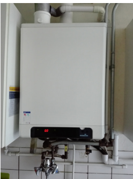
Fig. 1.2.3: Student 2: CV ketel Student 3: placed in storage
