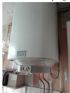
Fig. 1.2.5: Student 4: Electric boiler
