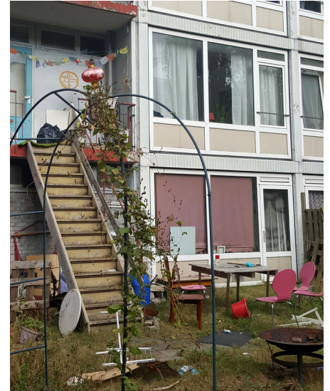
Figure 1.5.63 lack of maintenance (student group)
