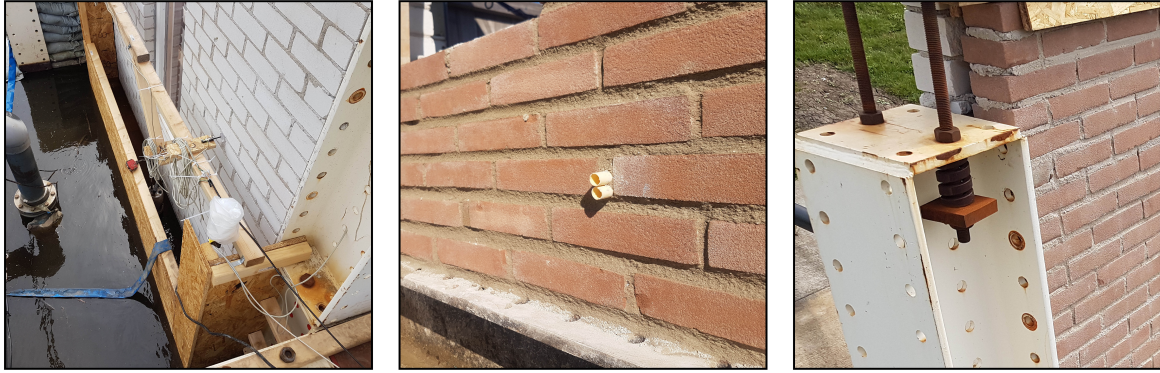
Figure 3.8: Left: The catchment box during testing. A small pump located inside the box is used to empty the box when needed. Centre: The small pipes used to mimic the weep holes. Right: location of the springs.
