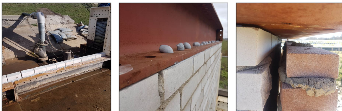
Figure C.4: Left: the first course of calcium silicate bricks. Centre: two-component epoxy glue at the top of the wall. Right: Existing gap between the steel beam and the clay wall.
