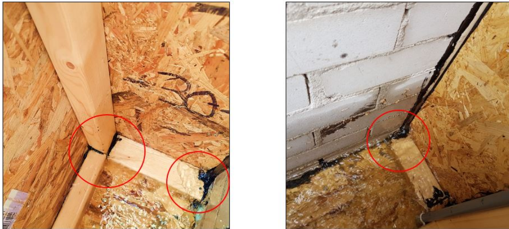
Figure 4.8: Photographs of the box leakages at the bottom of the box. In the corner three beams connect insufficiently; forming a pathway for the water to enter the box. At the locations where the box meets the steel rig also water was observed. It was tried to seal these points, but the water came through anyway.
