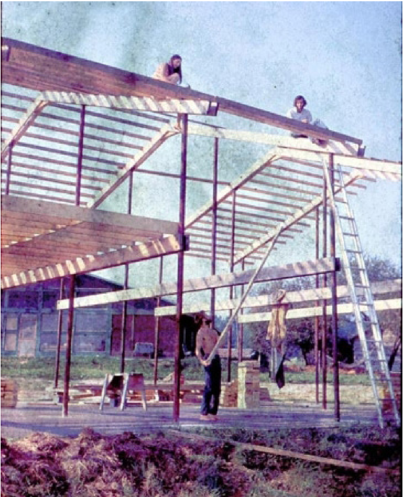
Figure 13. Construction of roof framework in Twin Oaks Community, 1960s. (Photo courtesy of Ray Jesse Blatt)
