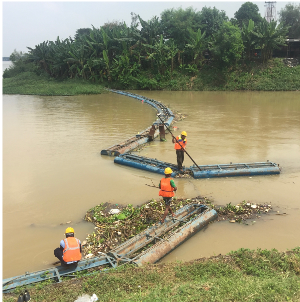
Figure 47: Workers let solid waste through floating retention boom before Mlirip Sluice (Mojokerto)
