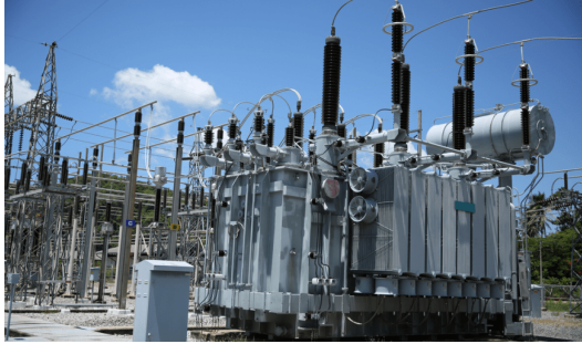
Figure 2.4: In service power transformer [16]
