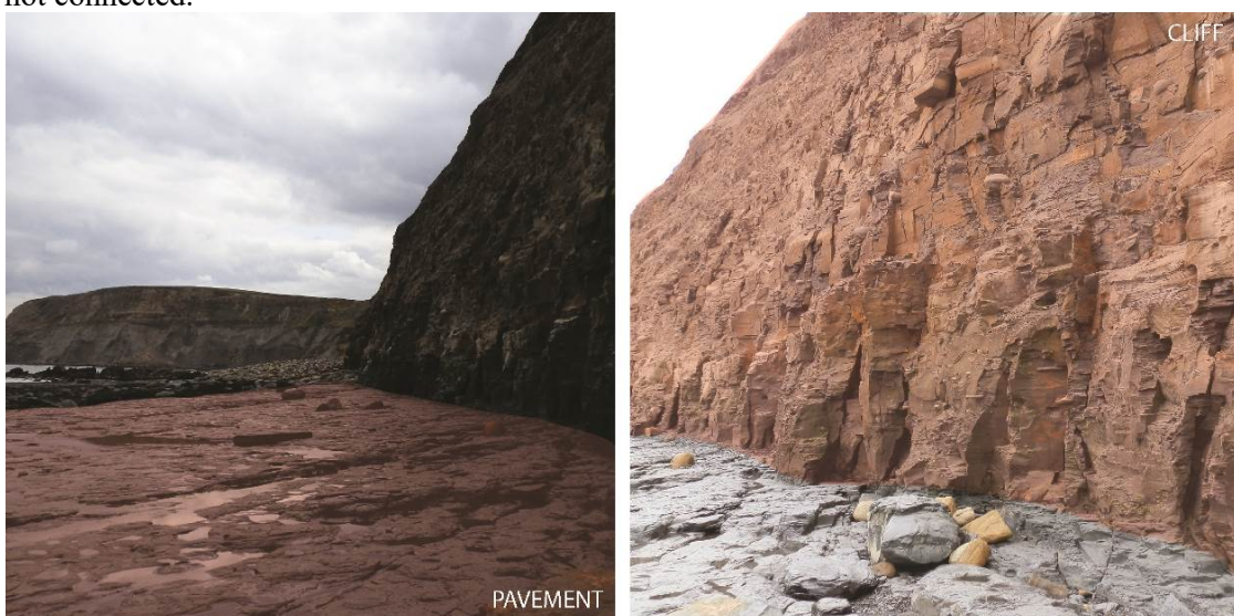
Figure 1 Pictures of the fractures in the pavement and cliff at the coast near Pore Mulgrave (UK).
