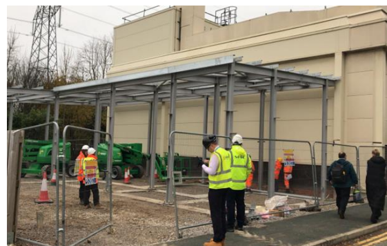
Figure 4. The safety zone selected around the steel erecting work to be monitored and controlled.
