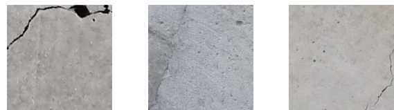
Figure 5: Example of cracked concrete images (Tomaszkiewicz & Owerko, 2023b)
