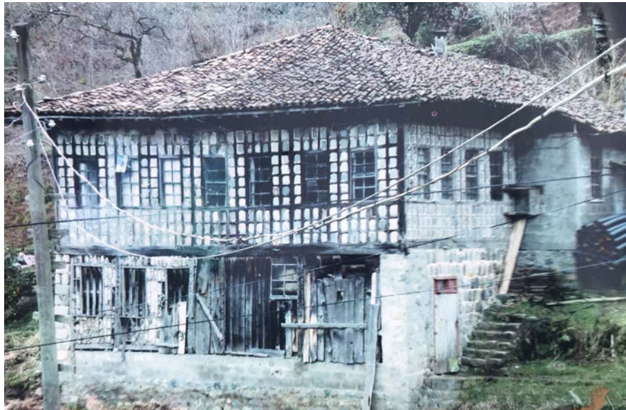
FIG. 4.8 Babalik mansion before its renovation already had some interventions done. Source: Family archives of Babalik mansion house.
