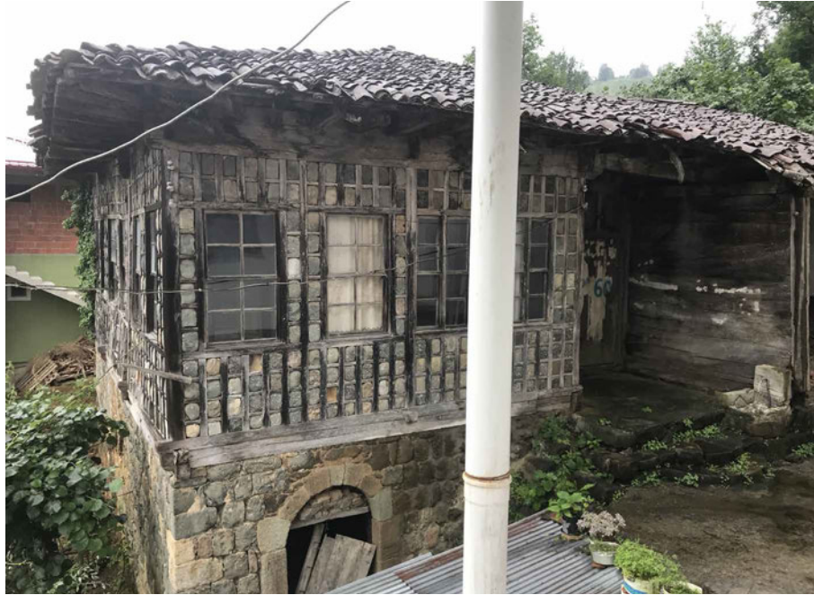
FIG. 6.6 The abandoned house due to inheritance issues.Source: author.
