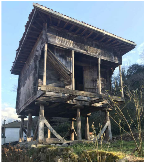
FIG. 4.3 A rectangular form of elevated storage house of the Okman family on wooden poles has eight wooden pillars with three on the opposite sides. Source: author.
