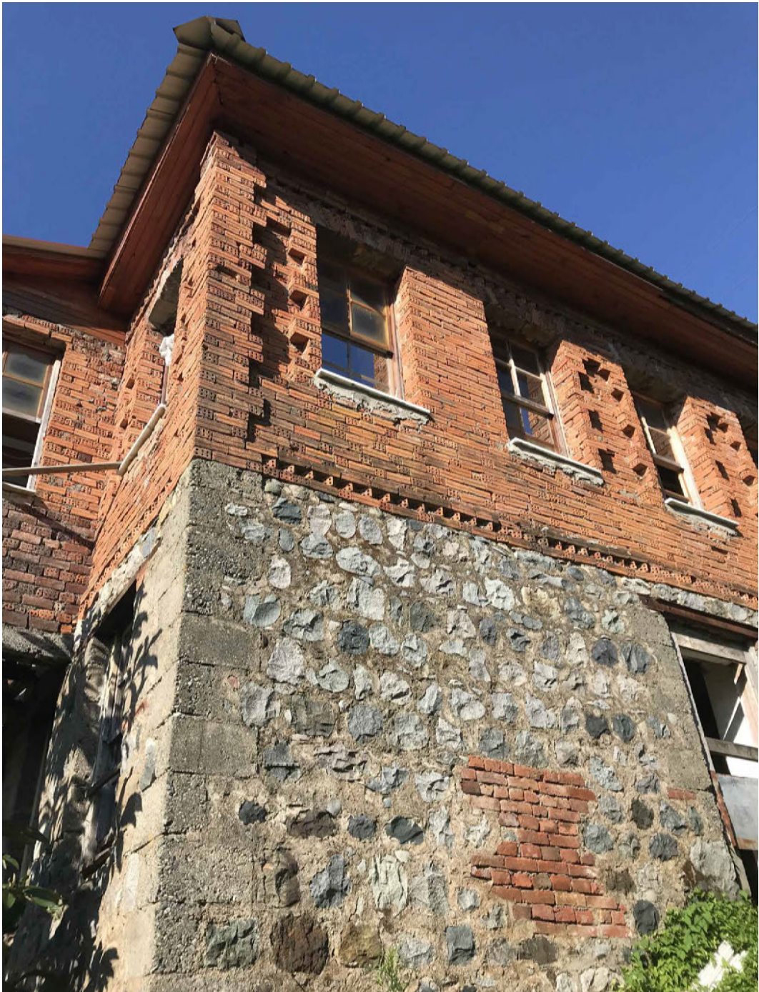
FIG. 6.20 The abandoned brick-built building was a recent building. Source: author.
