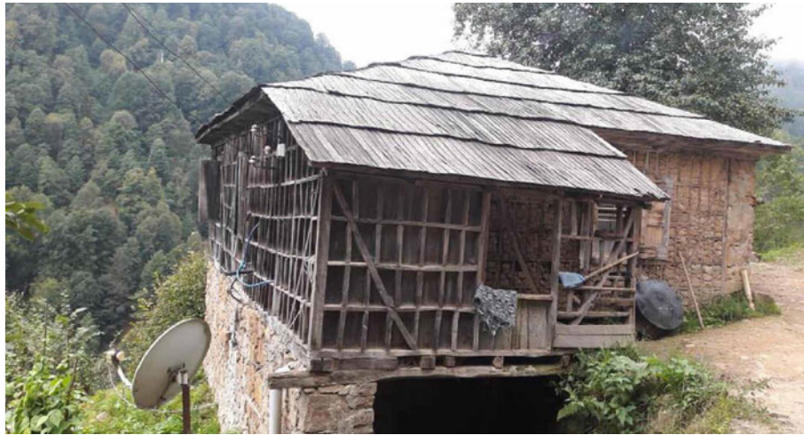
FIG. 3.21 Block-wooden technique extinct in the coastal part still exists in more inaccessible inland areas. 359 The thin, long, and narrow wooden slabs known as hartama are either used as roof tiles or as a support to roof construction laid under the roof tiles. Source: İsa Karaca Yeşilpınar Köyü, Yağlıdere / Giresun. Facebook Giresun köşe bucak https://www.facebook.com/giresunkosebucak/photos/
