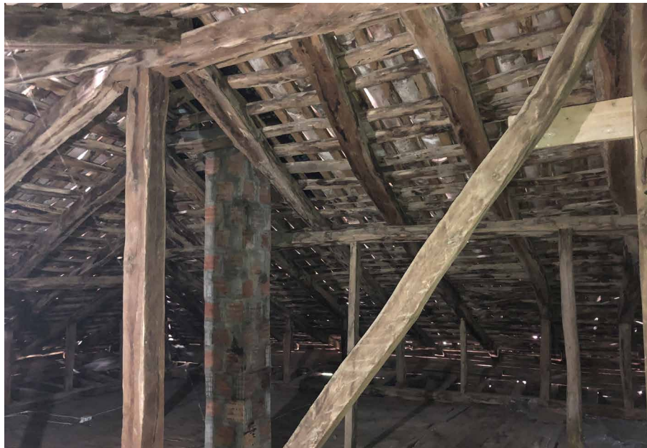
FIG. 4.16 Underneath the roof construction, there are pillars and trusses. The wooden boards are laid on them. Source: author.
