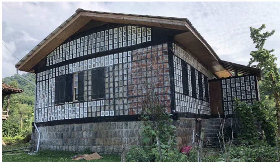
FIG. 6.19 The fast deterioration of the traditional vernacular buildings. Source: author.
