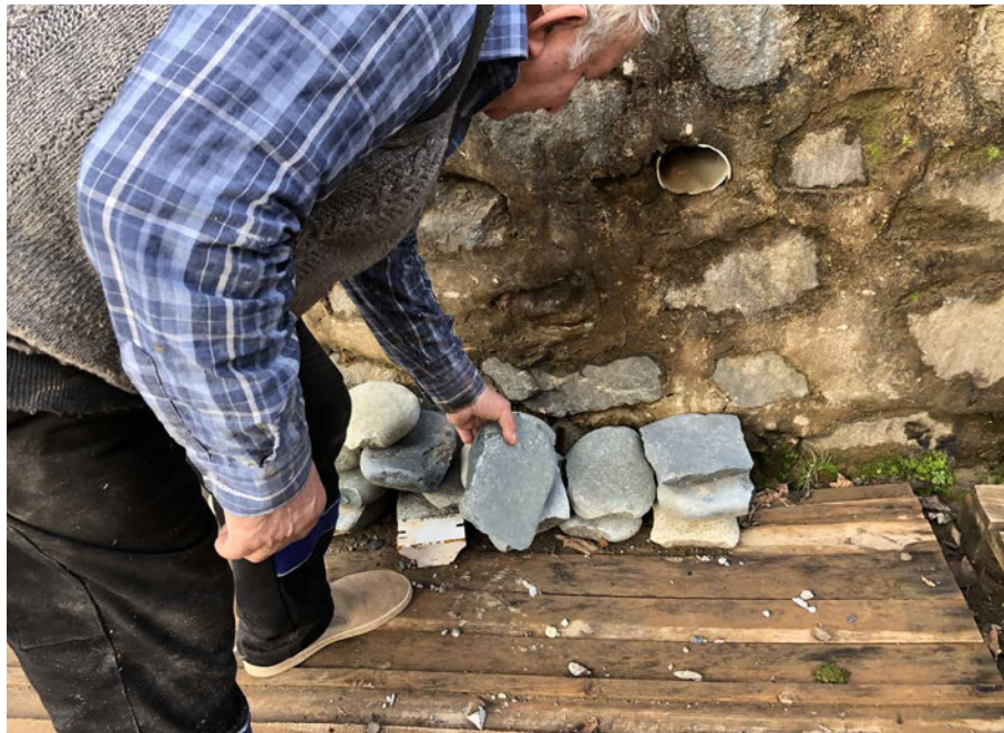
FIG. 4.9 The local stonemason Ş.S. shows the sizing of the stones used in the construction of cell-filling used in the construction. Source: author.
