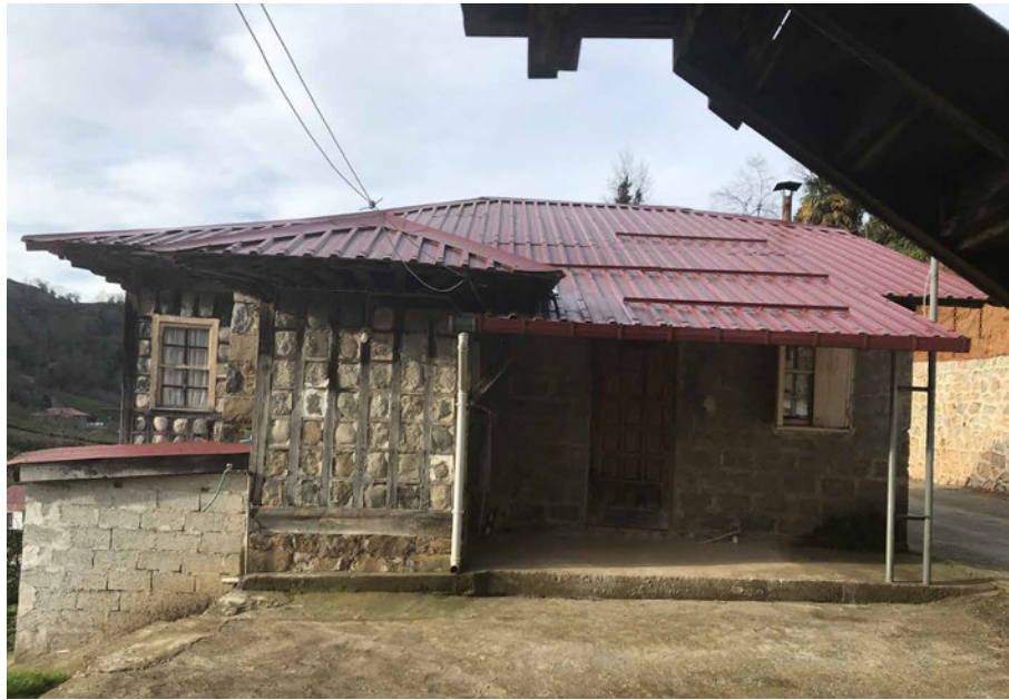
FIG. 6.7 An example of a maladaptation from a building with a metal roof construction as opposed to the traditional roof of hartama . The arc-like roof curve and detailing have disappeared with the change of material. The roof cover does not allow air circulation and solar gain anymore due to the material change. Source: author.
