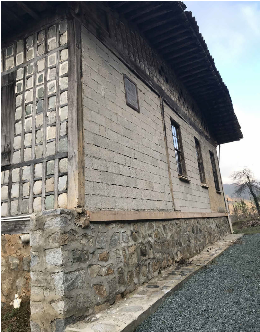
FIG. 5.20 The degradation of the rear façade of the Şevket Atac House due to landslides in Çağlayan Village in Fındıklı of Rize. Source: author.
