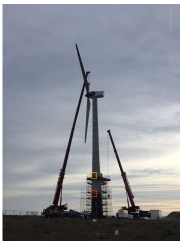
(a) Placement sensors
