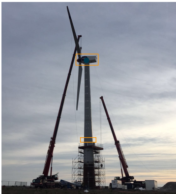
(a) Placement sensors
