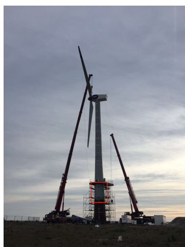
(a) Placement sensors
