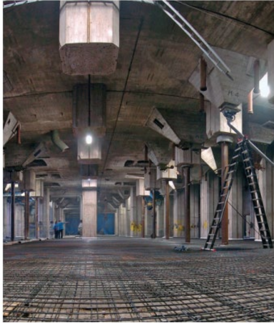
Figure 7: Square concrete columns have been partly replaced by slimmer steel columns (Debets, 2004)
