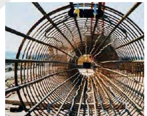
Figure 35, Geothermal pile with heat exchanger tubes attached to the reinforcement to be incorporated in the concrete (Parriaux, 2009)
