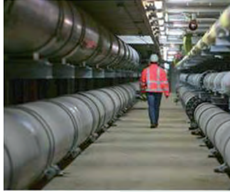
Figure 39, Utilidor in Amsterdam under the Mahlerlaan (Photo: H. Admiraal)
