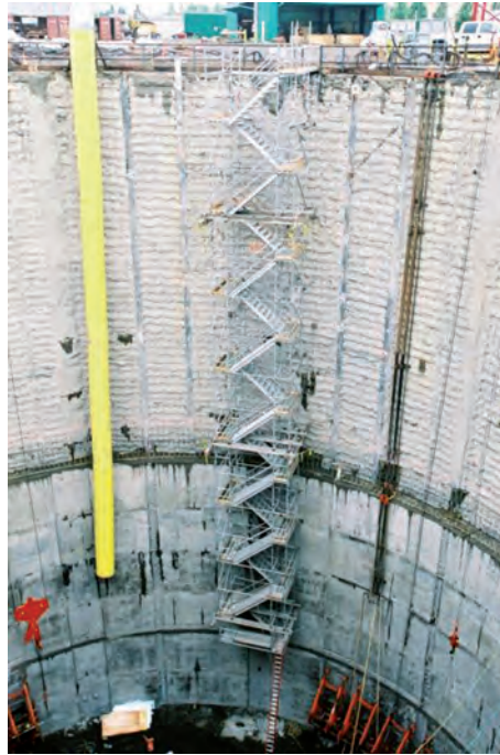
Figure 30, Deep Pump Station, Portland, Oregon, US
