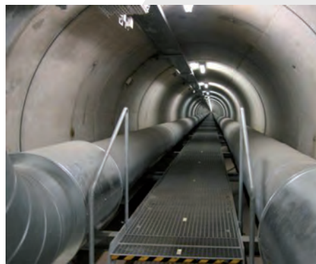
Figure 34, District Heat Tunnel in Cologne, Germany
