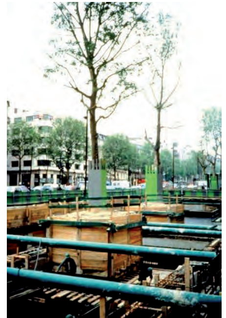
Figure 65, Maintaining trees during the construction of an underground car park, Champs Elysees Avenue, Paris
